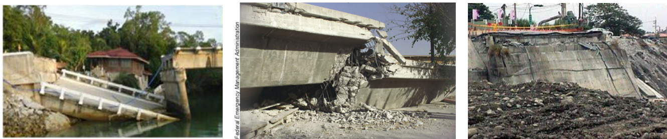
Figure 1. Some failure modes of bridge abutment
